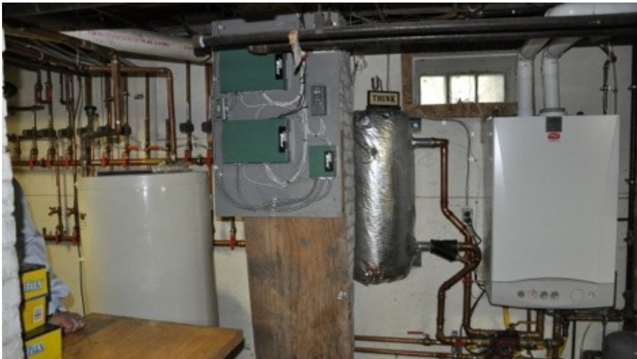
The mechanical room, with wall-hung boiler at right, thermal storage tank at left, and zone valve relays in the center.
